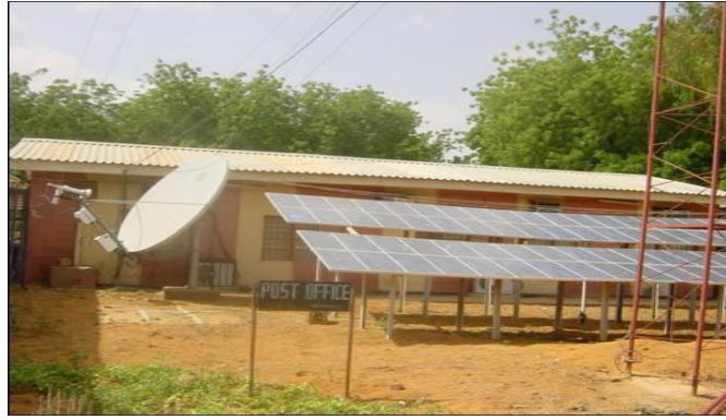
Fig. 7. Solar PV Internet Back-up at Nunet, UDU, Sokoto. [27].
