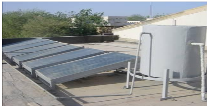
Fig. 8. Community Based Pilot Water Heater, UDUTH. [27].
